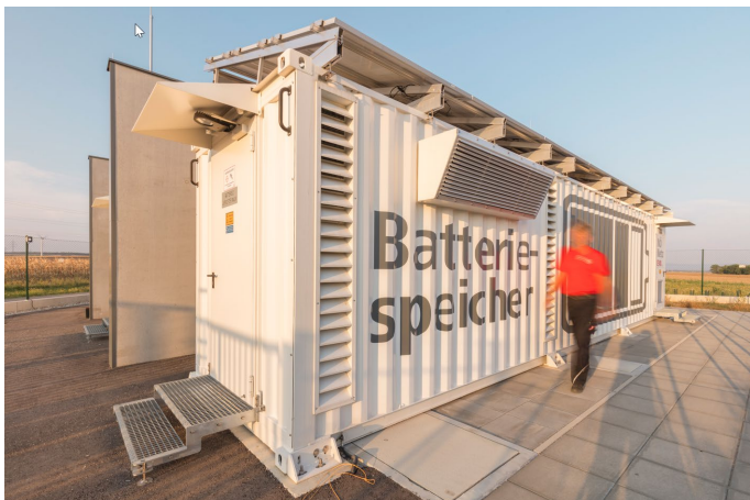
Utility-scale battery storage
