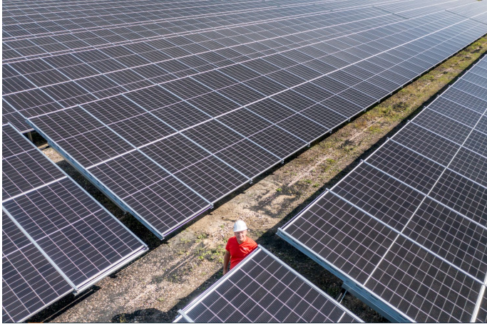
Large-scale PV plant
